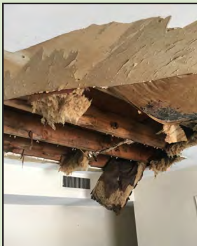
Water damage and mold.
