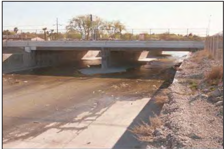
Clark County flood control facility. Source: BEC files.
