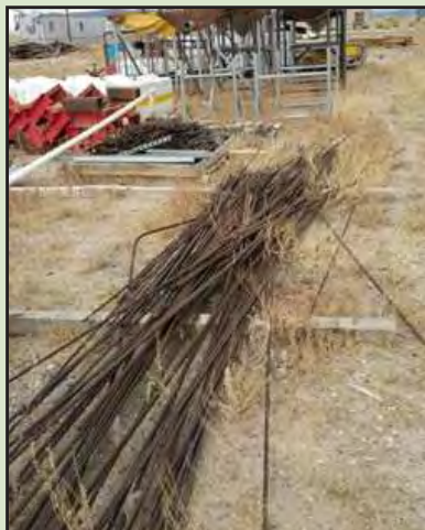
Rebar stored in stockpile area in southeast portion of fenced yard. Source: BEC files.
