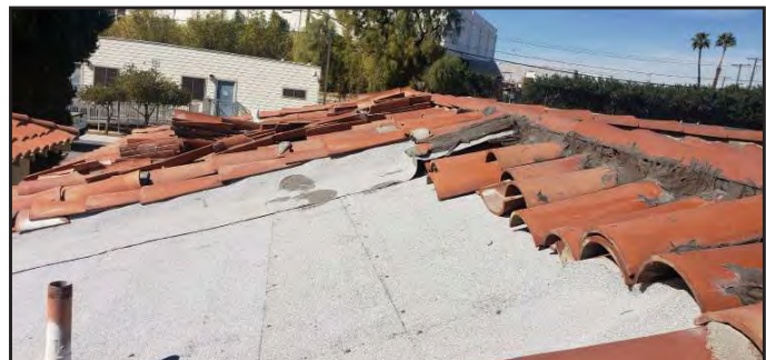
View of the subject building roof being surveyed and sampled for asbestos-containing materials prior to demolition.
