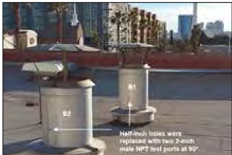
Exhaust stacks for Boilers 1 and 2.
