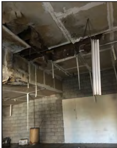
Damaged interior of Patriot's Plaza garage.
