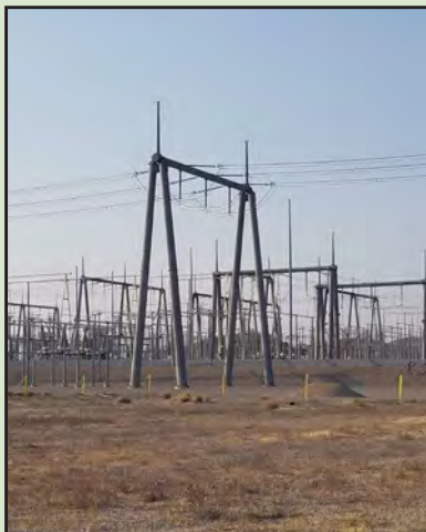
Existing Crystal Substation.
